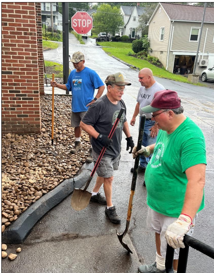
Pictured (left to right): Pat Hewitt, George Gamble, Rob Minnich, and Tim Gooch placing river rock around the foundation of St. Peter's Church Saturday, August 12 th to replace outdated landscape features.
